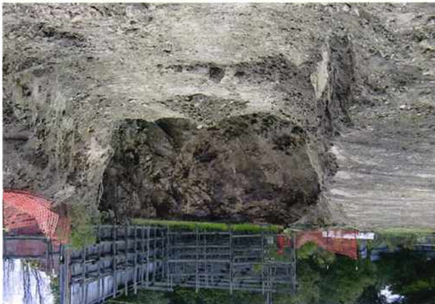
Photo No. 1 View of over-excavation facing east from west end of ramp
