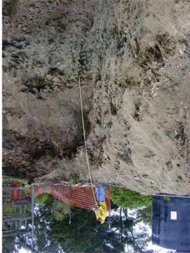
Photo No. 2 View of stained soil on north wall of over-excavation at approximately 12 feet below ground surface
