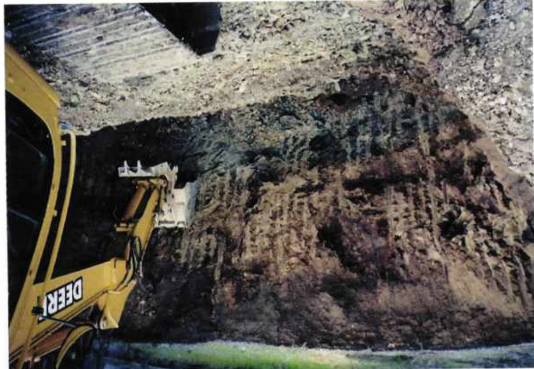
Photo No. 3 View of east wall when stained soil was first encountered
