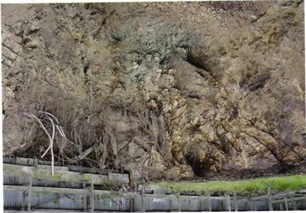
Photo No. 4 View of stained soil left in place in the southeast corner of the over-excavation
